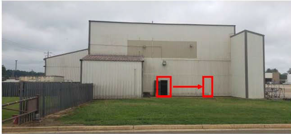
Figure 22. Image showing the current composition of the northeast elevation. The door indicated in red would be replaced with a new single-leaf steel door and shifted in location to allow for a small addition to the mechanical room.
