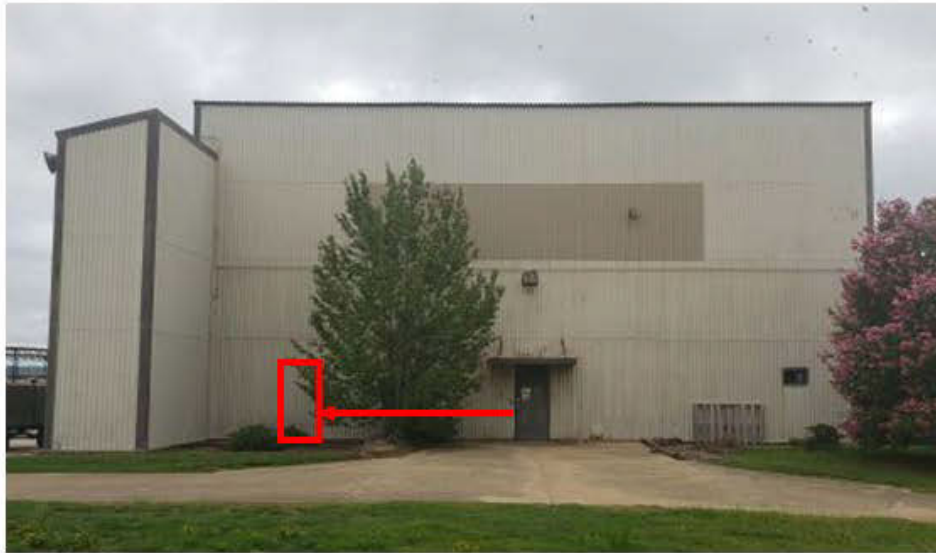
Figure 17. Image showing the current southwest (side) elevation. The door indicated in red would be replaced in-kind and shifted in location (indicated by red arrow and box). The bush located to the far right blocks the view of the addition from this image.
