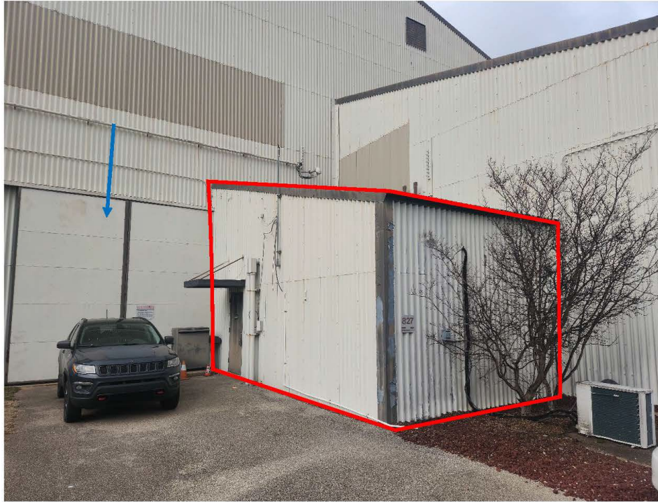
Figure 21. Detail showing the ca. 1980 addition on the rear elevation indicated in red, which partially covered an existing door indicated by the blue arrow.
